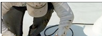
Left: A worker installs white roofing on an Atlanta school. Photo credit: Department of Energy.
